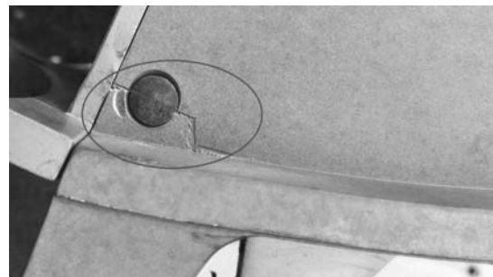
图7 “Z”字形裂纹 Fig. 7 Zigzag crack
